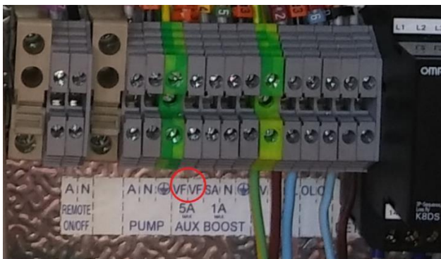
Picture of heat pump terminal strip
