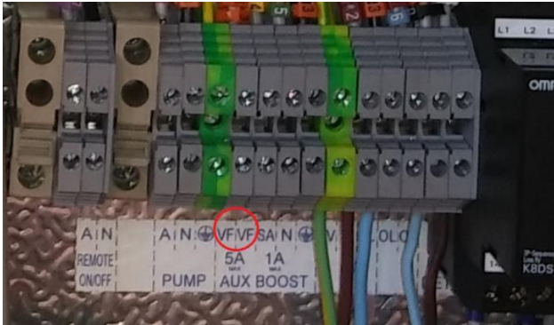
Picture of heat pump terminal strip
