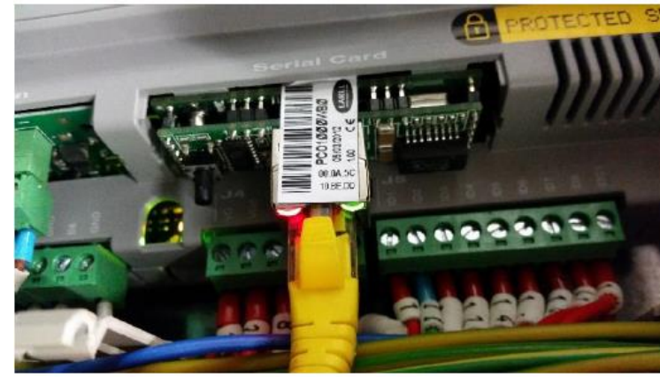
Status RED- card not communicating with heat pump Ethernet GREEN- Network connection OK
