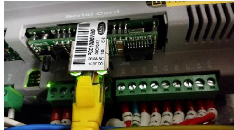
Status GREEN- card communication OK Ethernet GREEN- Network connection OK
