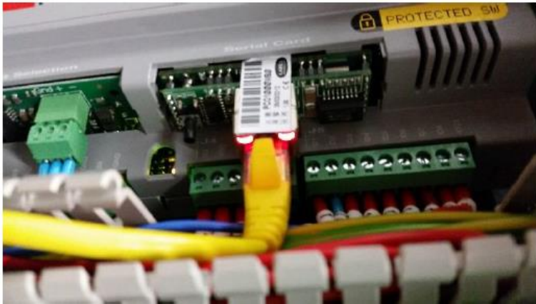
Status RED- card not communicating with heat pump Ethernet RED- No connection between card and network
